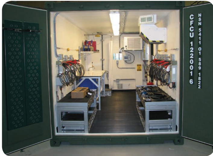
Shown above is the 20-Foot ISO Battery Maintenance Shop
