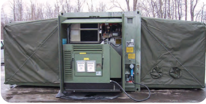
Rear of TMF showing generator
