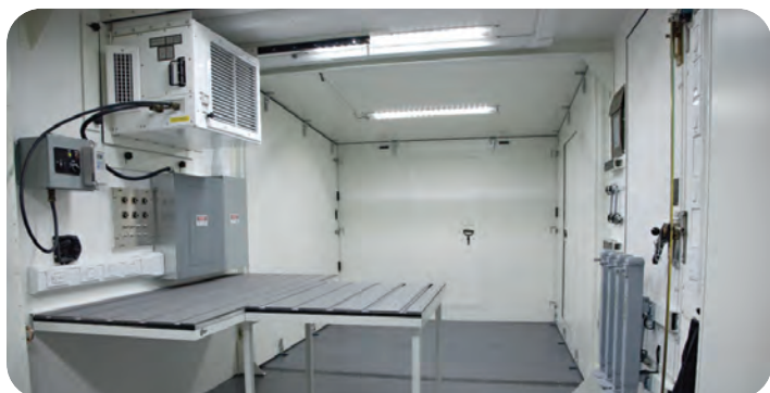
HESAMS shown with ECU, power distribution system, and work table
