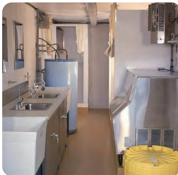
Medical Utility Facility
